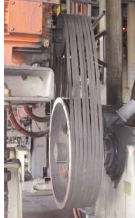
Original V-belt Drive
