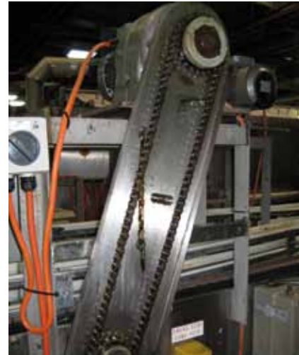
Original Roller Chain Drive
